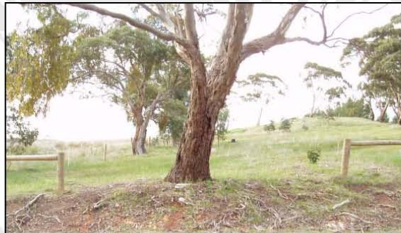
The same strut arrangement seen from the side. The strut holding the wires away from the tree is directly behind the tree. The wires are in place but can't be seen due to the light at the time the photo was taken.
